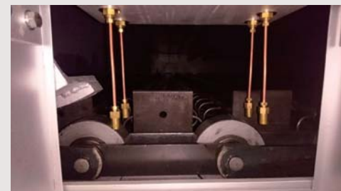
▲ Automatic lubrication point
